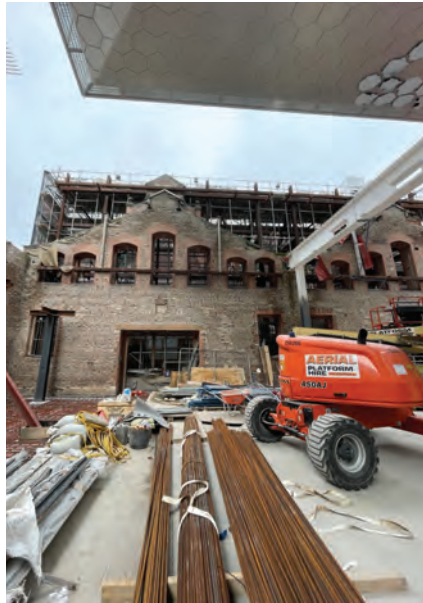
View of Block 2 structural frame under construction. Photograph taken from Block 2 ground level
