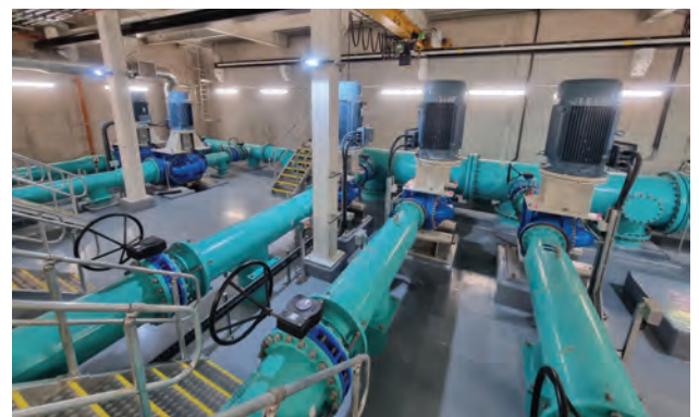
Lee Road Water Treatment Plant interior
