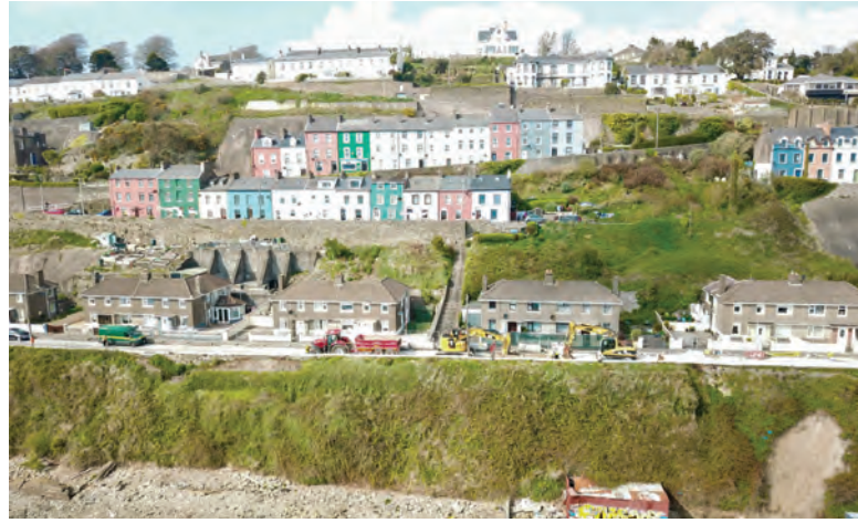
Construction of a Ø750mm gravity sewer at depths of up to 5mBGL along an embankment above the harbour. The topography of the catchments as well as the condition and age of existing buildings and retaining structures were a particular challenge on this project
